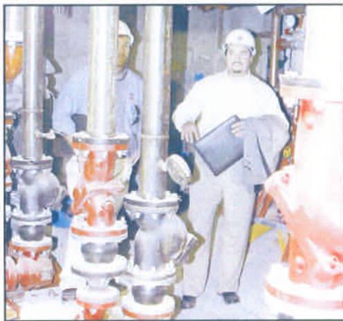
Reporter photo by Steven Furlow Matthew Mayol (right), an architect with the Odle McGuire and Shook Corporation, and co-worker Ben Griffin (left) show off water pipes and other maintenance capabilities in the expansion of the Lebanon Public Library Wednesday evening, during a tour for library board members and staff.
